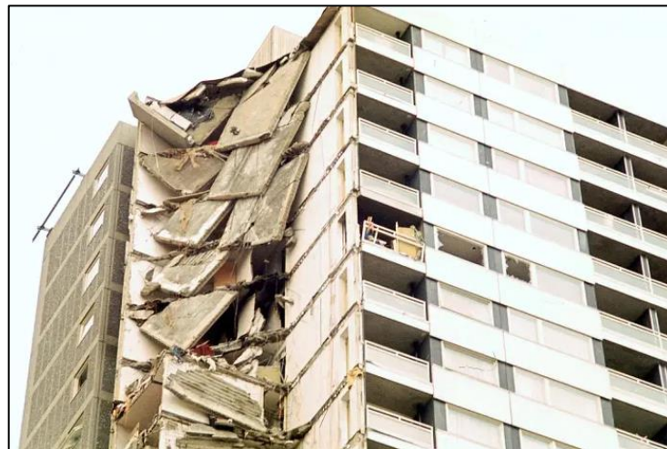
Figura 2.1 – Colapso parcial do Ronan Point Apartment Tower.
