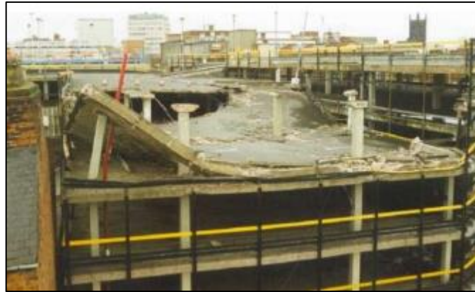
Figura 2.12 – Colapso parcial do Pipers Row Car Park.
