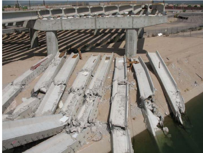
Figure 35 – Collapsed beams, (OESTERLE et al., 2007)
