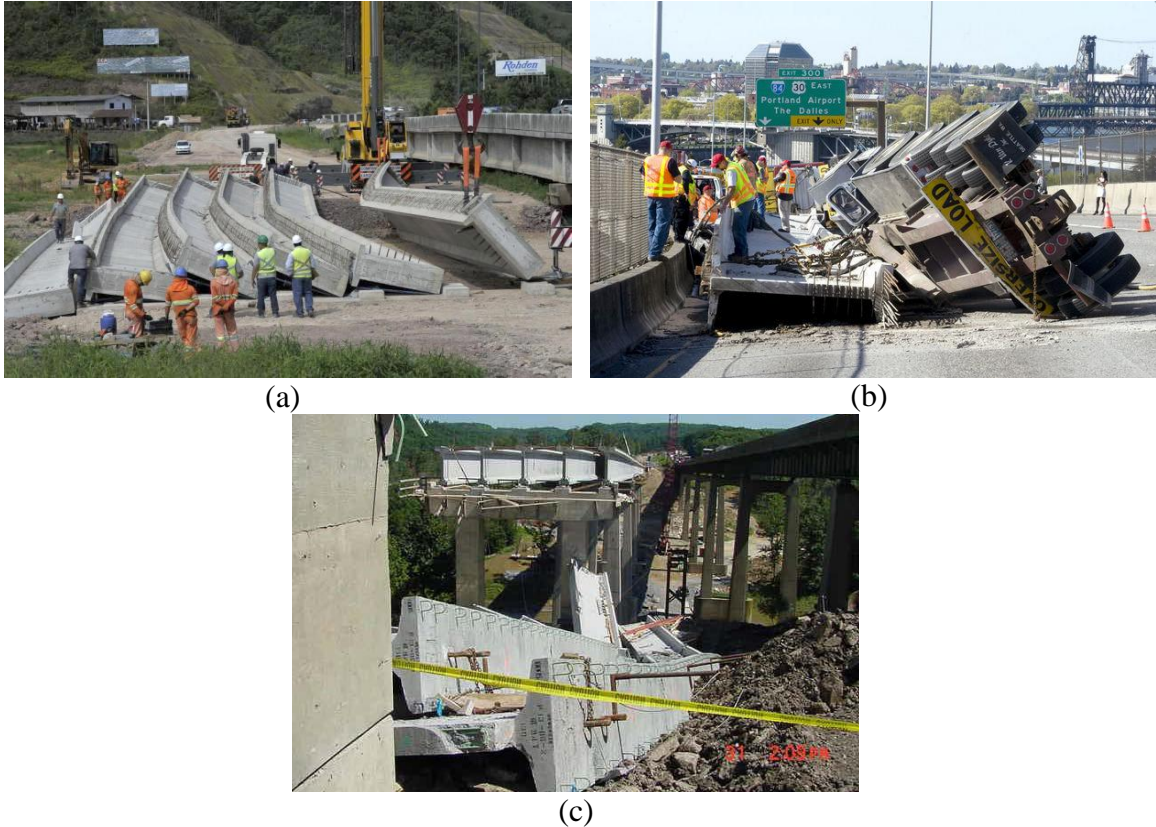
Figure 26 – Accidents occurred during transitory phases of construction
