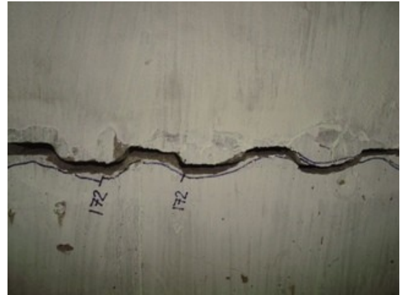
(b) Fissura na interface
